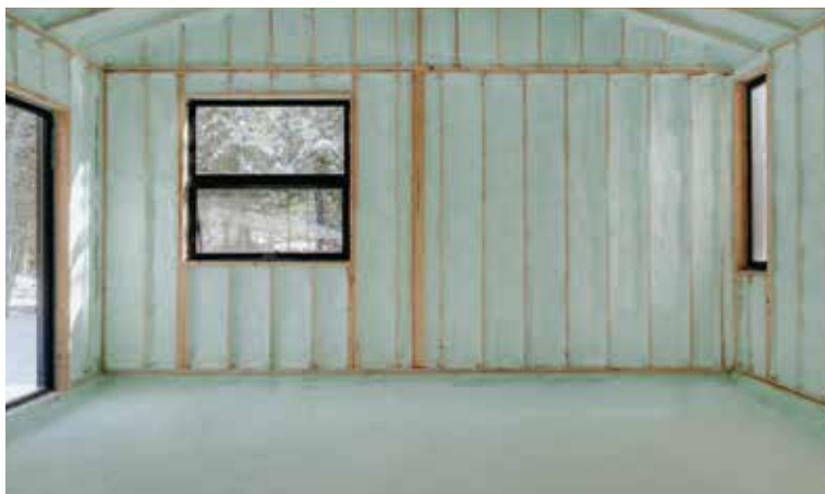
Slab on grade project with roof, walls and slab insulated with Heatlok Soya HFO.
