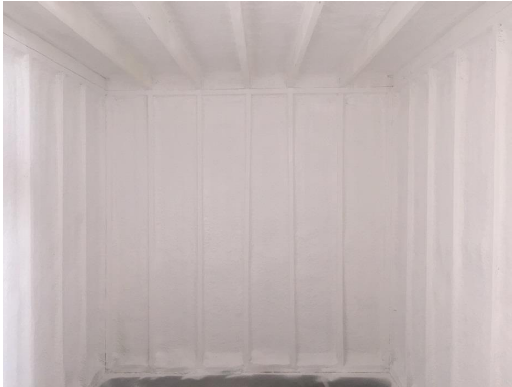
Figure 2. Example of application where the product (white) serves as the thermal barrier over MD spray urethane cavity insulation (and overexposed studs/joists) (1) in wood-frame basement walls and ceiling.
