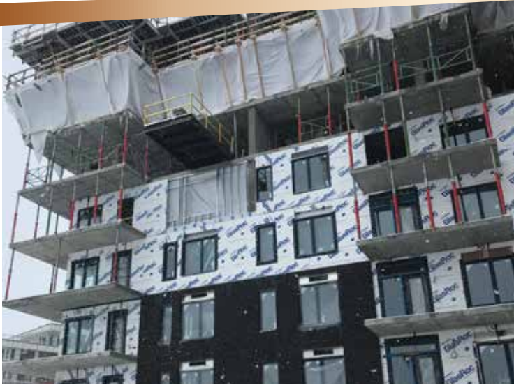
Example of productivity of the D-Max system. The cladding is installed from the ground floor to the third floor, the interior insulation is installed on levels 4 and 5 and the structure is poured on levels 6 and 7.
