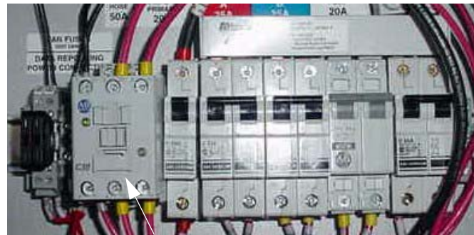
C30 Contactor Assembly Installed
