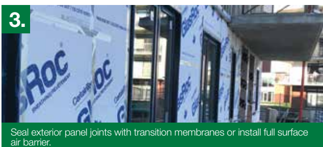
Installation of exterior sheathing on Z-bars and mineral wool in front of slabs and columns.
