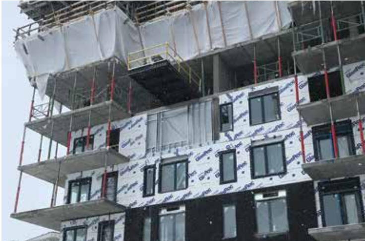
Example of productivity of the D-Max system. The cladding is installed from the ground floor to the third floor, the interior insulation is installed on levels 3 and 4 and the structure is poured on levels 6 and 7.
